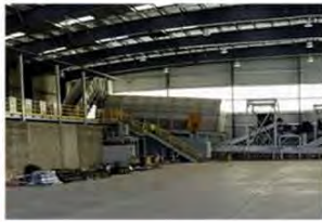
Organics Receiving Facility - ORF
