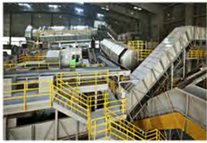
Material Recovery Facility - MRF
