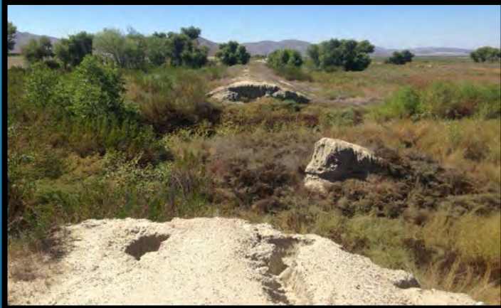
Breached Levee Looking West (opening over 100ft wide)
