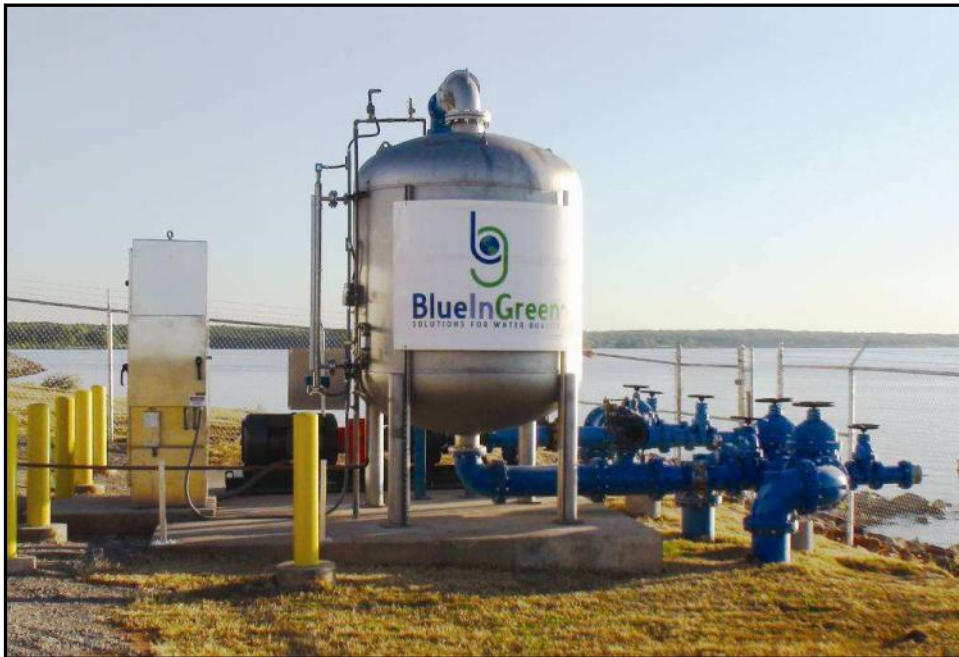
Figure 22: BlueInGreen SDOX Installation at Lake Thunderbird, OK
