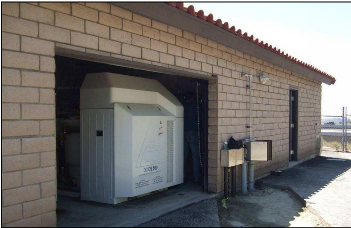
Figure 24: Oxygen Generator Installation at Oso Reservoir in Mission Viejo, CA
