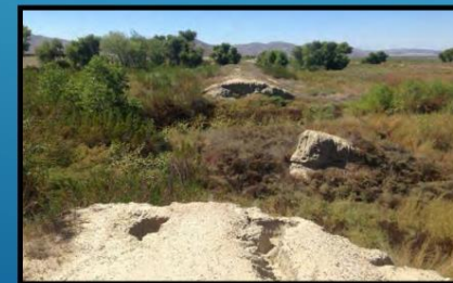
Breached Levee Looking West (opening over 100ft wide)
